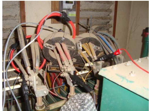
Figure 4 - Data Logger is connected to the Bus-bar for Load Measurements
