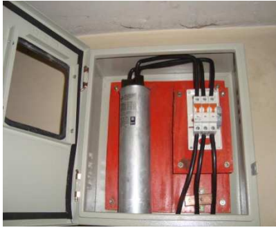
Figure 2 - Installed Capacitor at MAV Substation.
