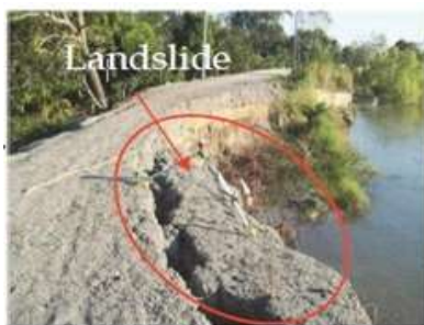
Figure 3: Occurrence of piping and landslides at river bank
